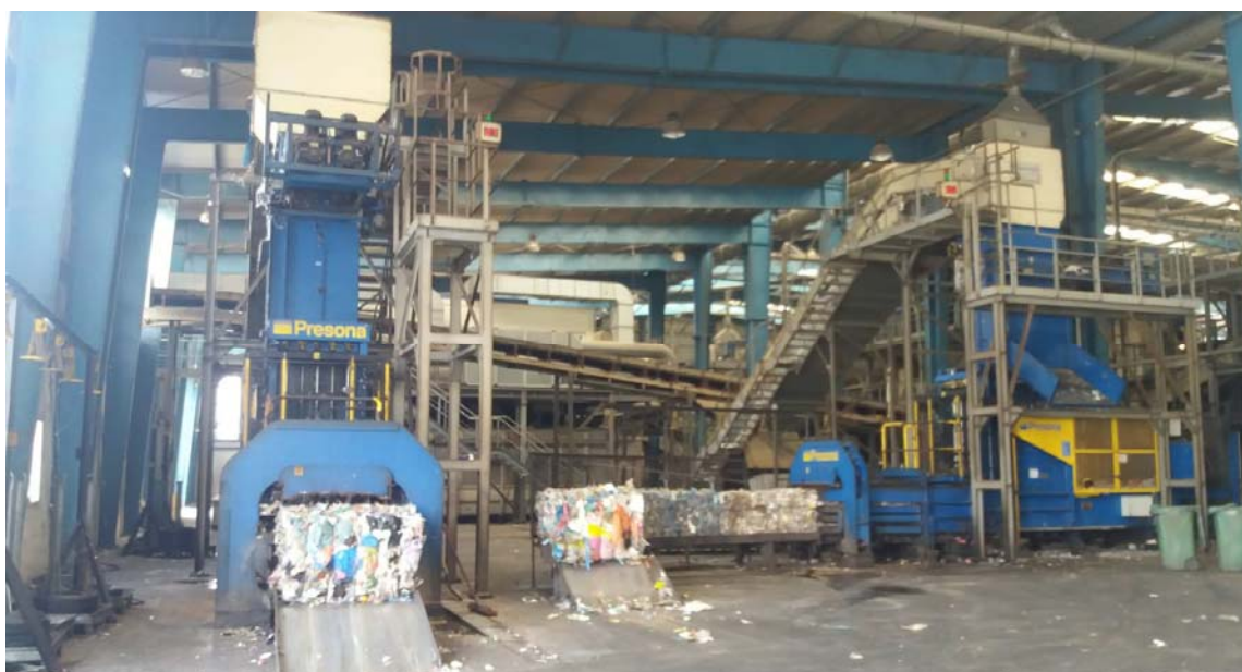
Figure 3: Mechanical Separation Facility
